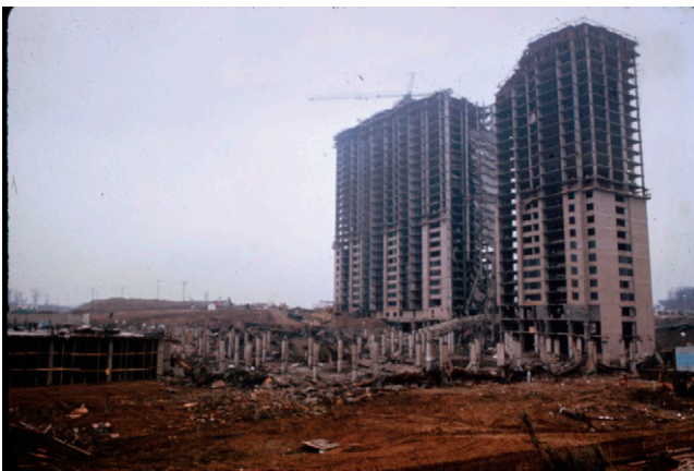
Fig. 3. Another view of the collapsed structure (courtesy of NIST)
